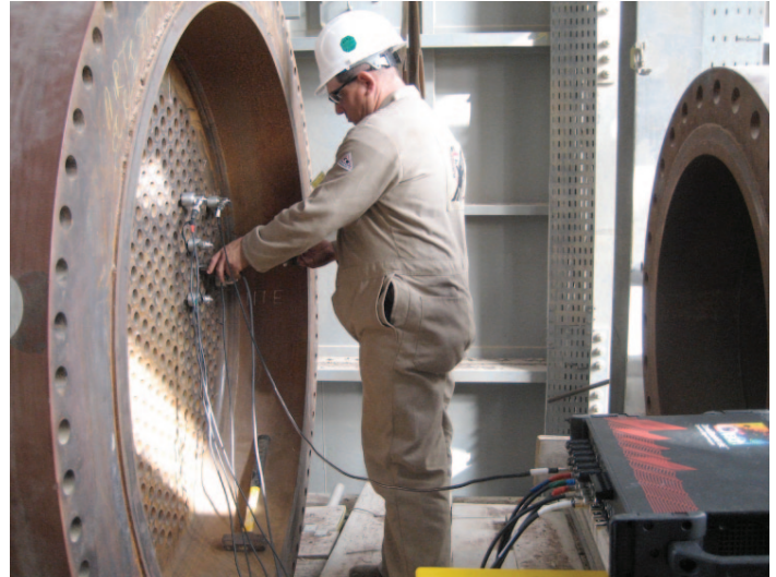
Figure 5: Example of connection of transducers for frequency response on heat exchanger
